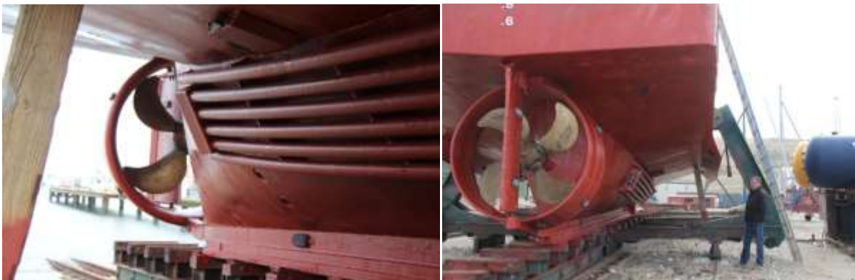
Figure 30. Cooling system is in a wrong position, disturbing water flow through the ducted propeller; efficiency of the propeller decreases quickly.
