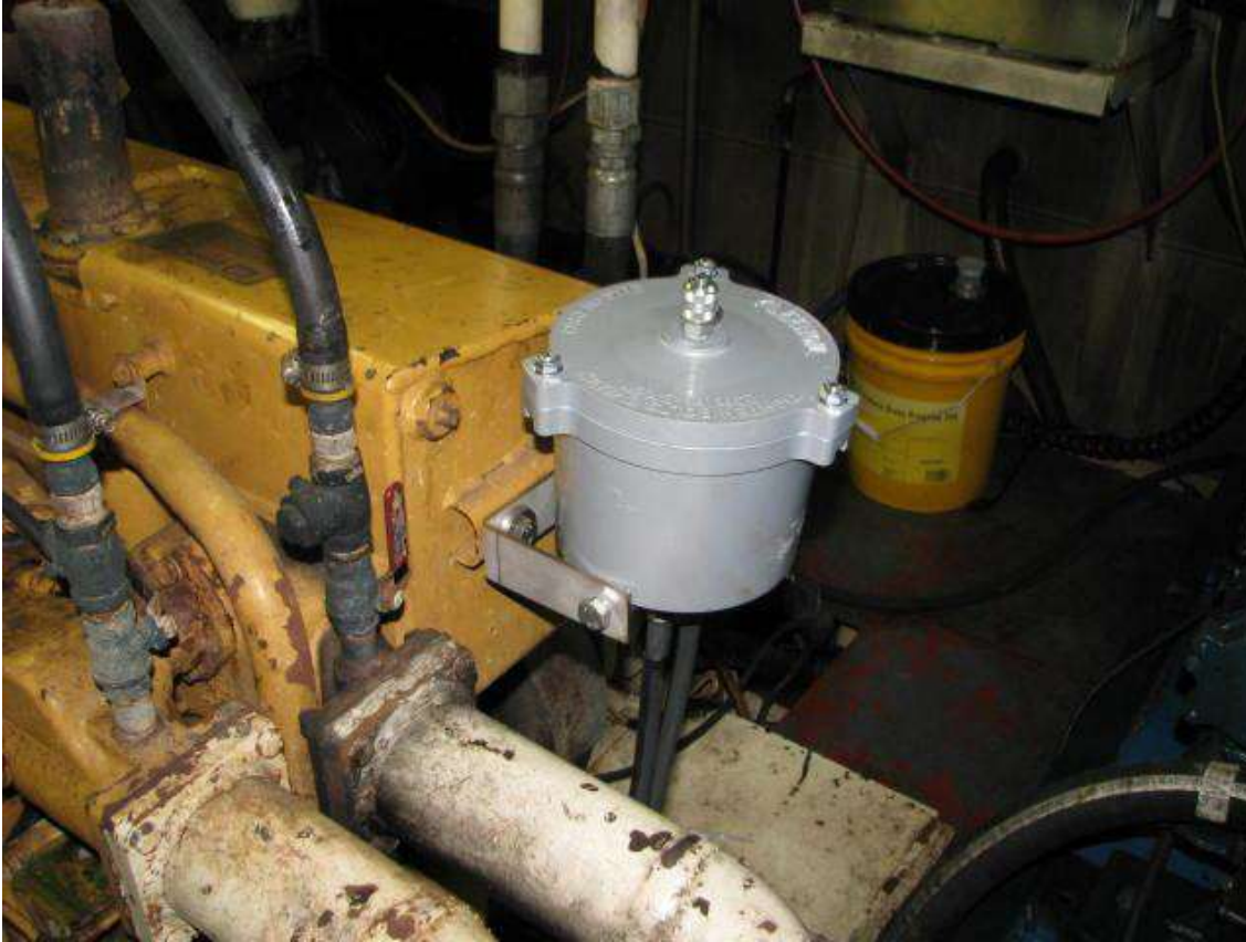
Figure 49. By-Pass Oil Filtration System
